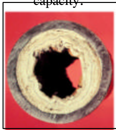
Figure 11.8: A pipe with accumulated mineral deposits. The cross section clearly indicates the reduction in pipe capacity.
